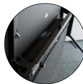
Kabelkanal cable duct
